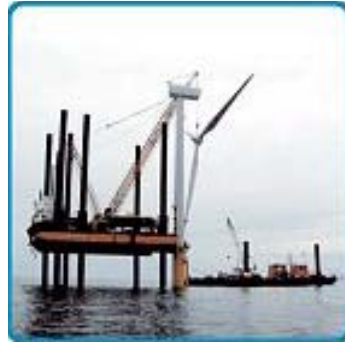
Blyth Offshore UK 4MW
